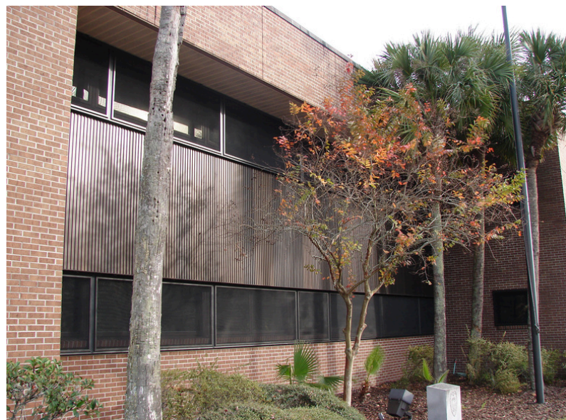
Precinct rear protected as well. Screens provided a solution across all windows.
